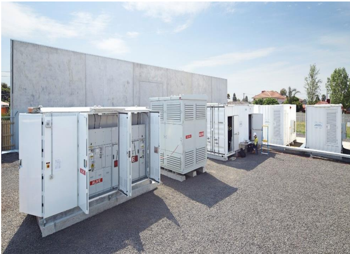
AusNet Services GESS facility. Image courtesy ABB.
